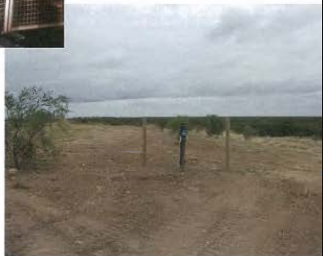
Deep wells installed to manage LFG emissions
